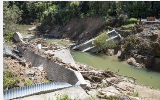
The bridge on No 4 Road washed out on 29 January 2023. Source: RNZ
