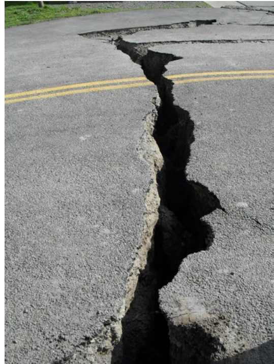
2010 Canterbury road rupture. Source: National Emergency Management Agency
