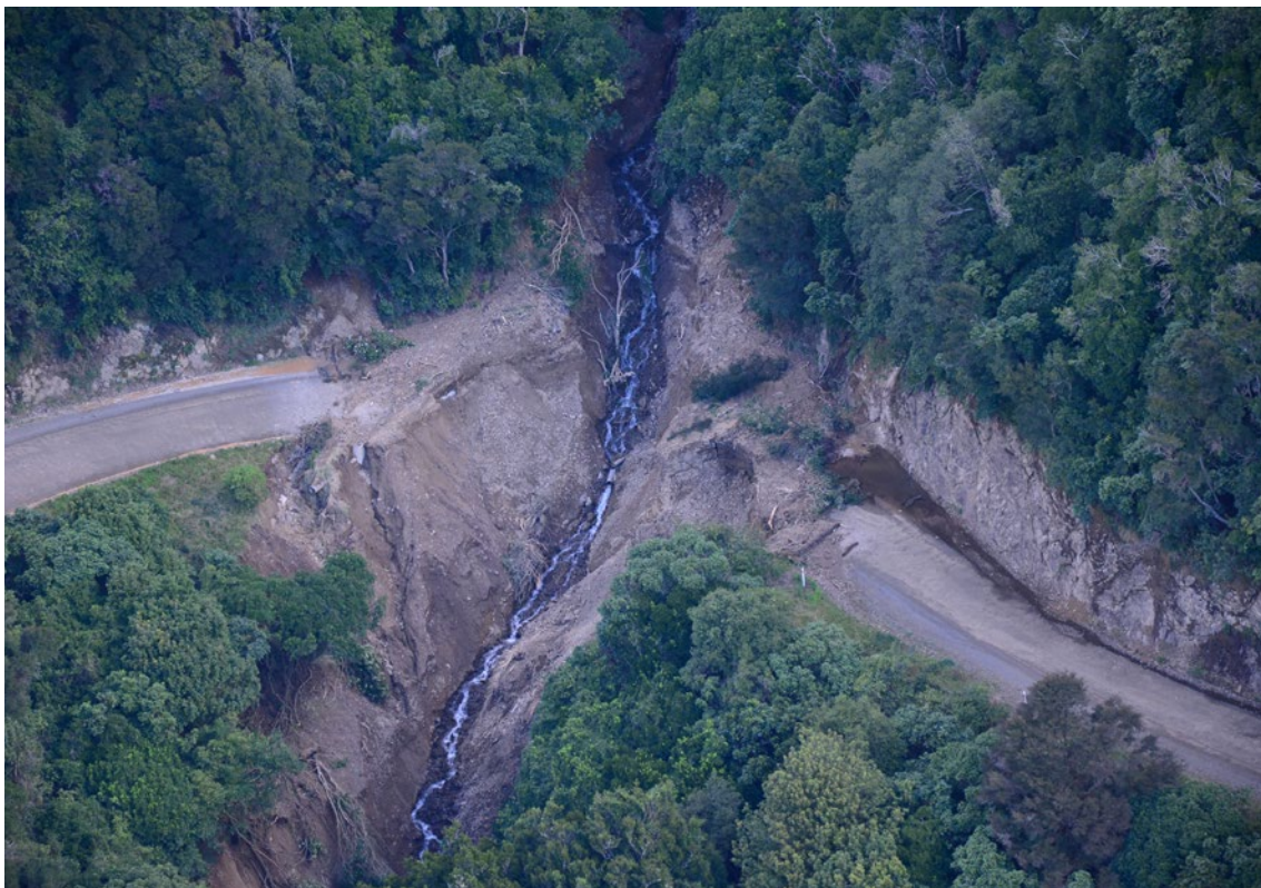
Damage to transport infrastructure - road washout caused by flooding, 2011. Source: Whakatāne District Council
