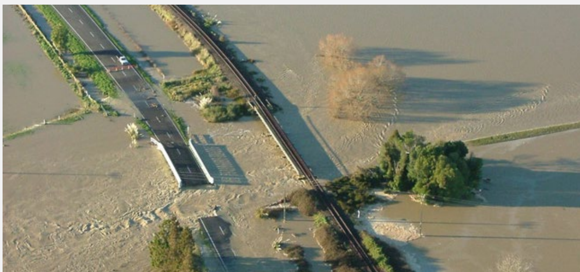
SH2 Reids Central Canal Bridge, Rangitāiki Plains 2004 Flood. Source: Bay of Plenty Regional Council
