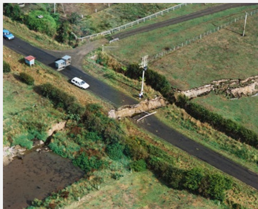
Edgecumbe earthquake main rift across McCracken Road. Source: GNS Science Photographer: Lloyd Homer
