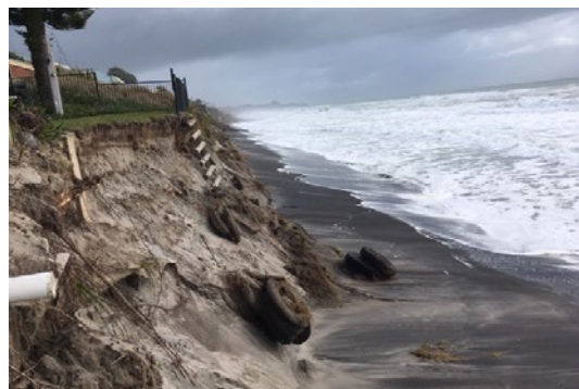
Erosion on beach accessway at No 183 Pukehina Parade, 2020. Source: Western Bay of Plenty District Council
