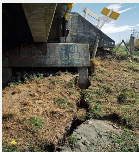
Damage from Edgecumbe Earthquake 2 March 1987. Source: GNS Science Photographer: Lloyd Homer
