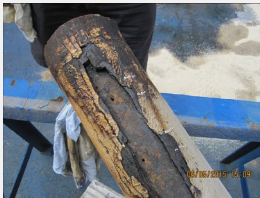
Damaged pipe after its removal. Source: Bay of Plenty Regional Council
