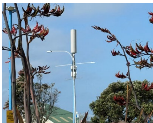
Telecommunications tower. Source: Bay of Plenty Regional Council
