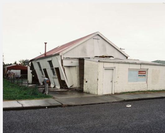
Building damaged by Edgecumbe Earthquake, 1987. Source: GNS Science Photographer: Lloyd Homer
