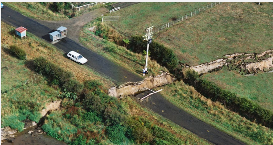
Ground cracking – 1987 Edgecumbe Earthquake. Source: GNS Science Photographer: Lloyd Homer
