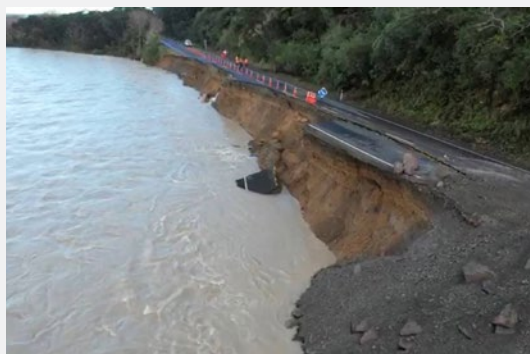
A section of SH35 near Te Kaha has collapsed into Motu River. Source: NZ Herald
